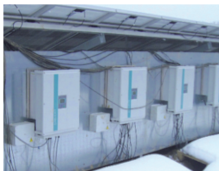
Messy installations cause safety risks and technical deficiencies.
